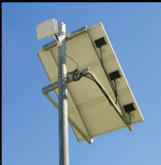
▲ SunWize PV system powering a SmartSensor HD
